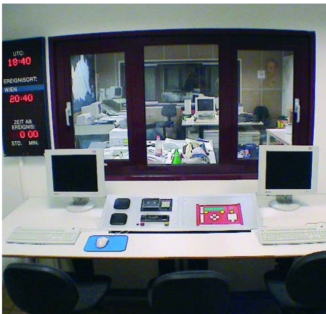
Main control centre
